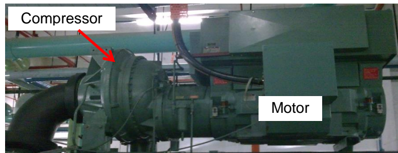
Figure 1.17 Photograph of an open-type compressor system
